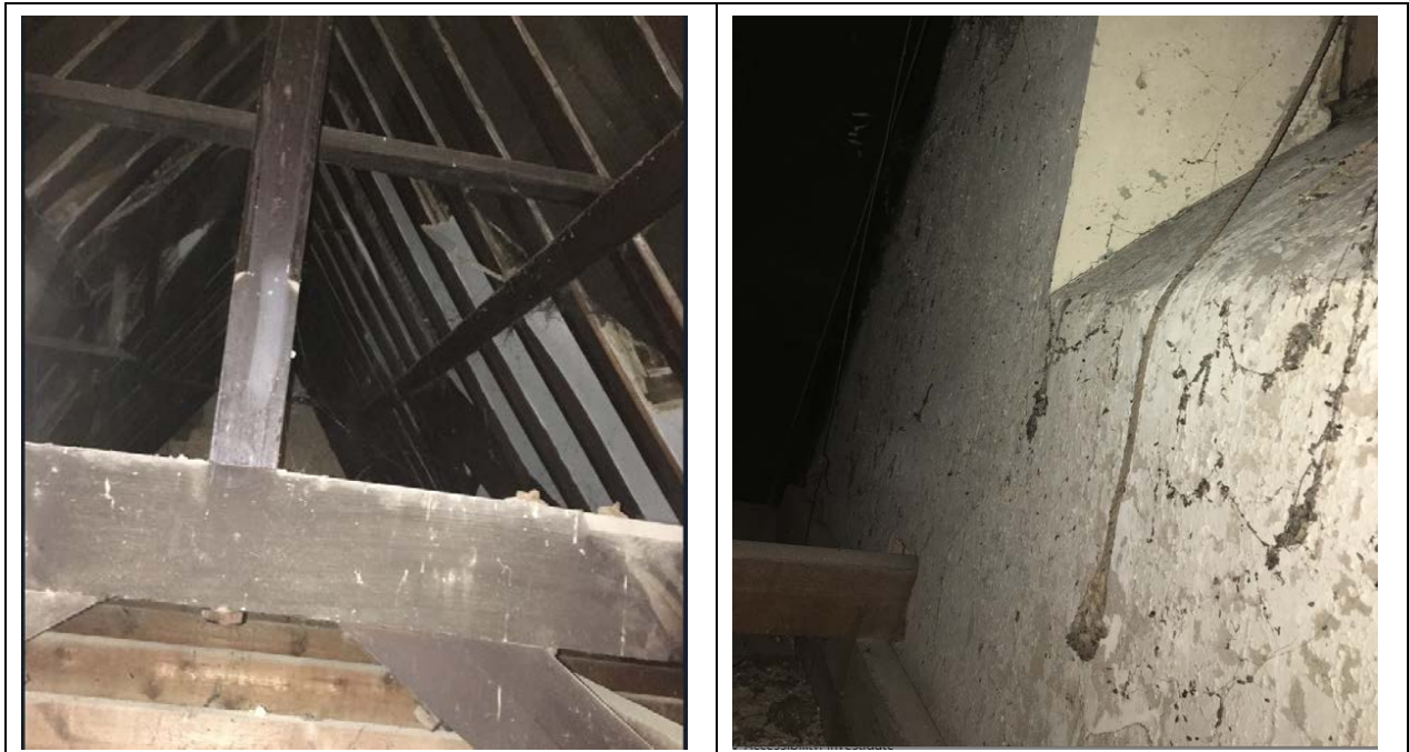
Figure 5 - Showing vaulted roof space and deteriorating plaster on gable end
