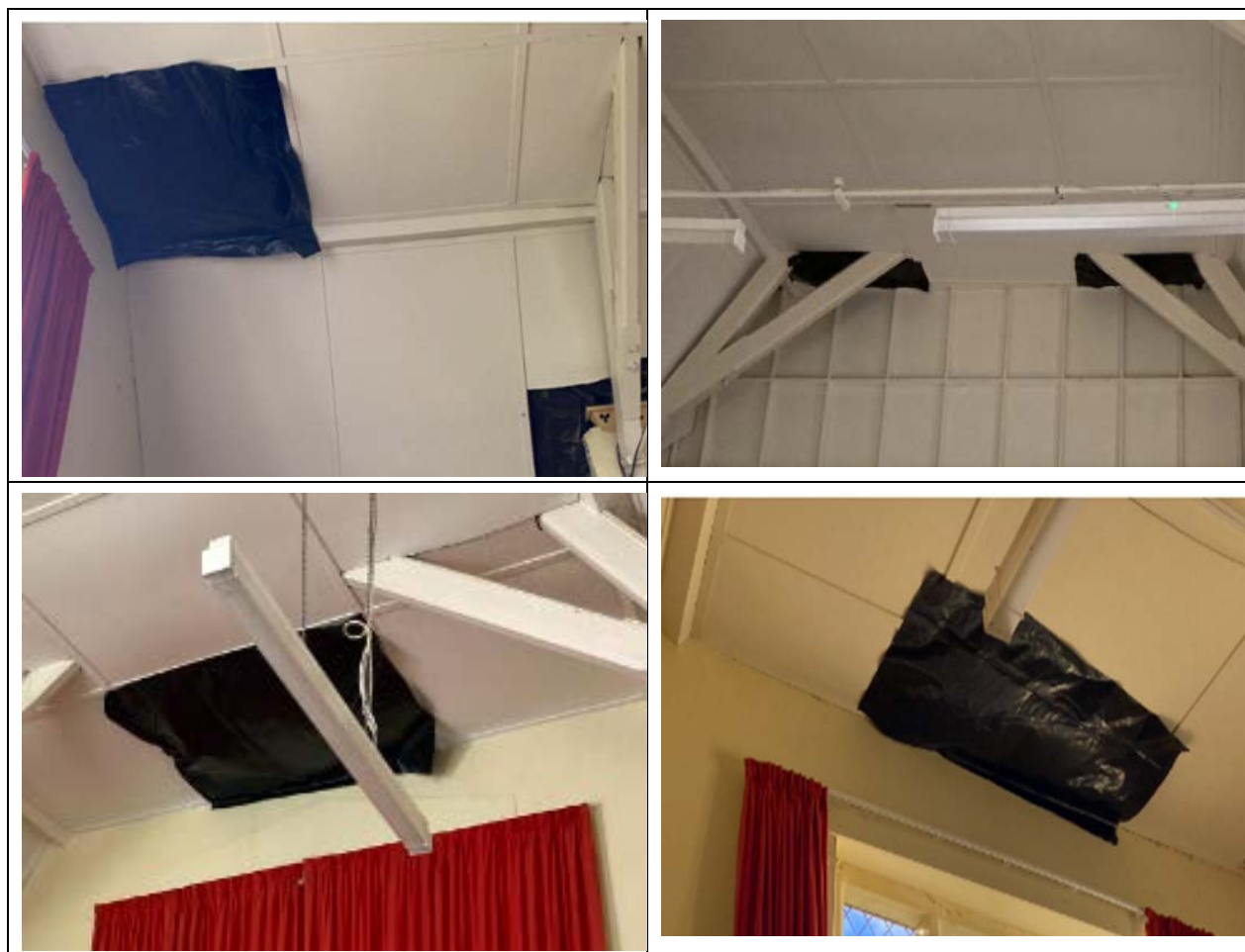
Figure 2 - Holes in Village Hall ceiling
