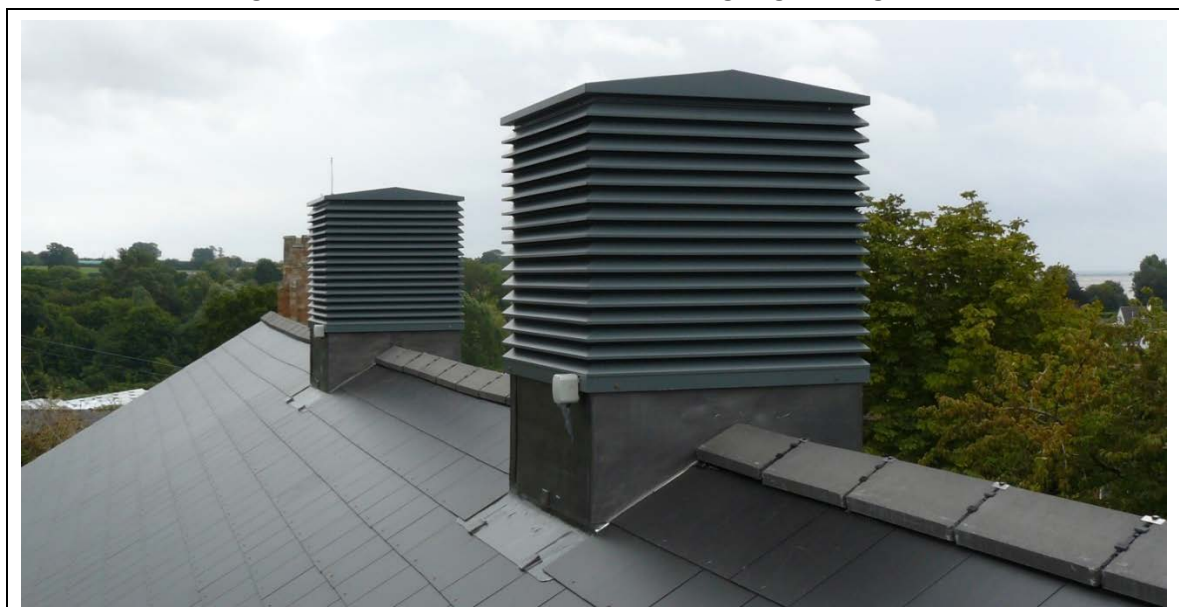
Figure 4 - Passive ventilation using turrets on Lymestone Village Hall
