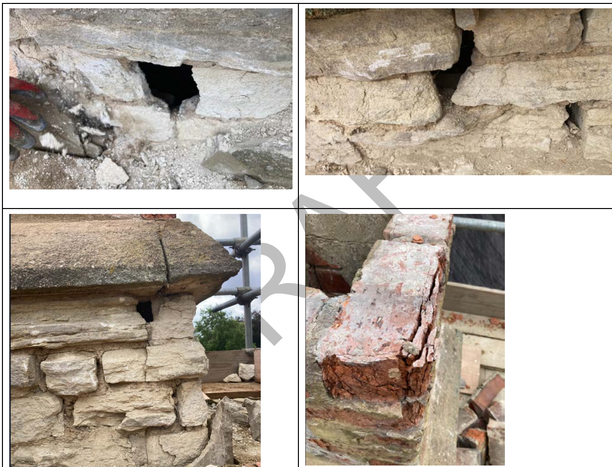
Holes and cracks in eroded stonework and shattered brickwork
