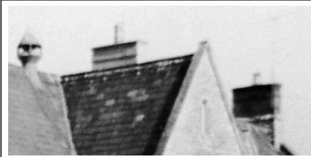
1950s photograph showing poor chimney pot replacement
